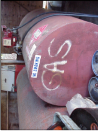
2. Gasoline tank in containment shed.
