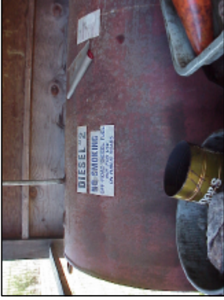
3. Diesel tank in containment shed.
