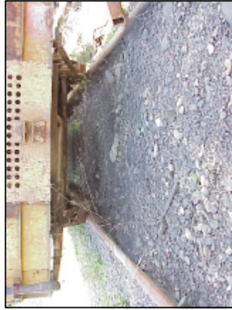
5. Oil beneath equipment on siderail.
